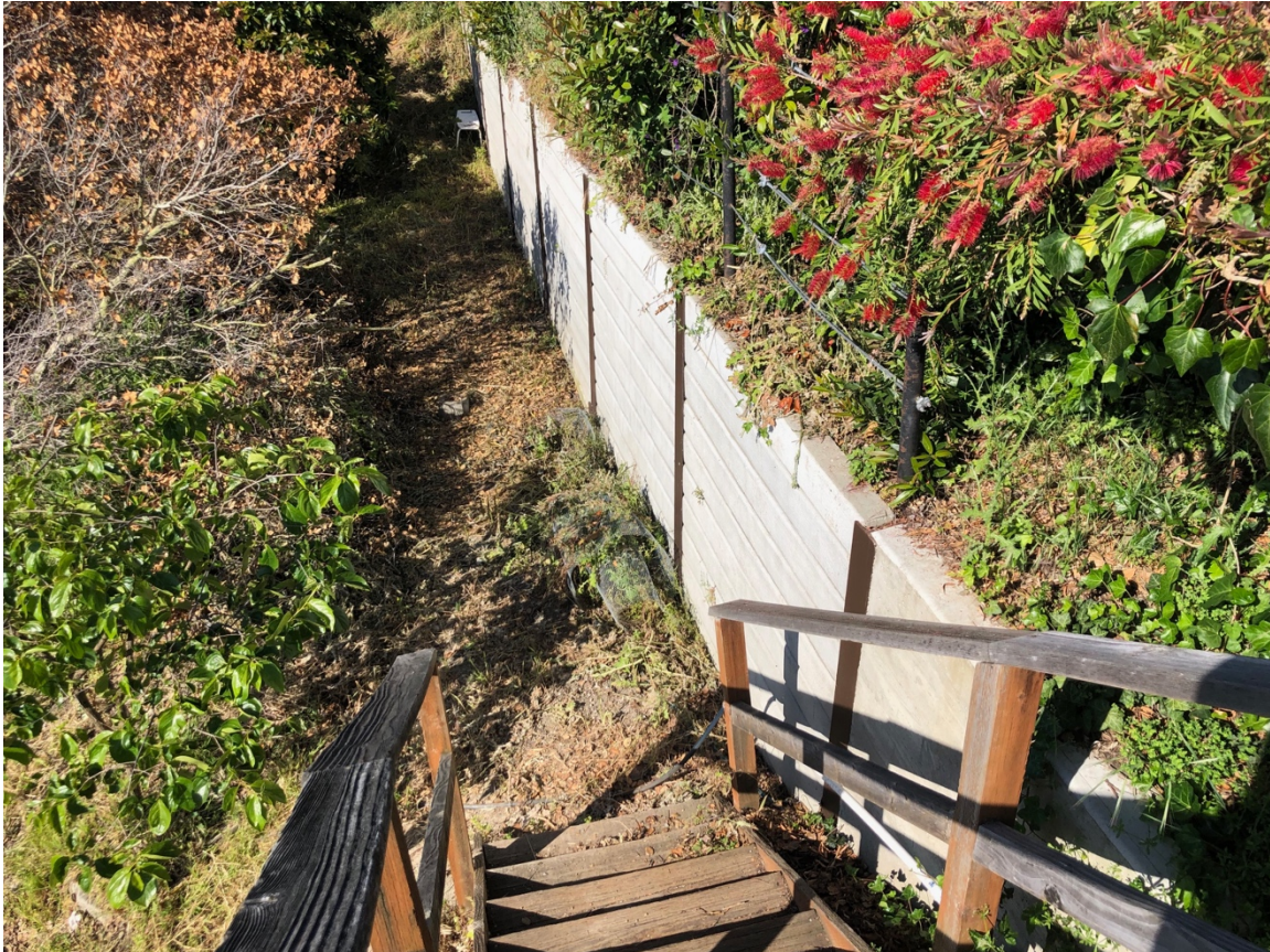
Photo 5: View towards the southwest of the I-Beam retaining wall along the rear of 2843 Arguello Drive that we understand was constructed over 35 years ago and also contains tie-backs that extend into the slope.
