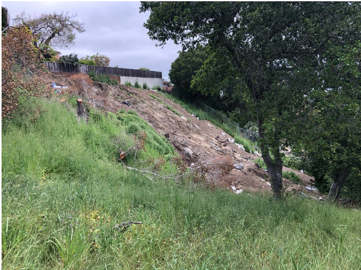
Photo 1: View towards the north of the affected slope along the rears of 2839 and 2843 Arguello Drive as it appeared after tarps were removed several days before the photo was taken.
