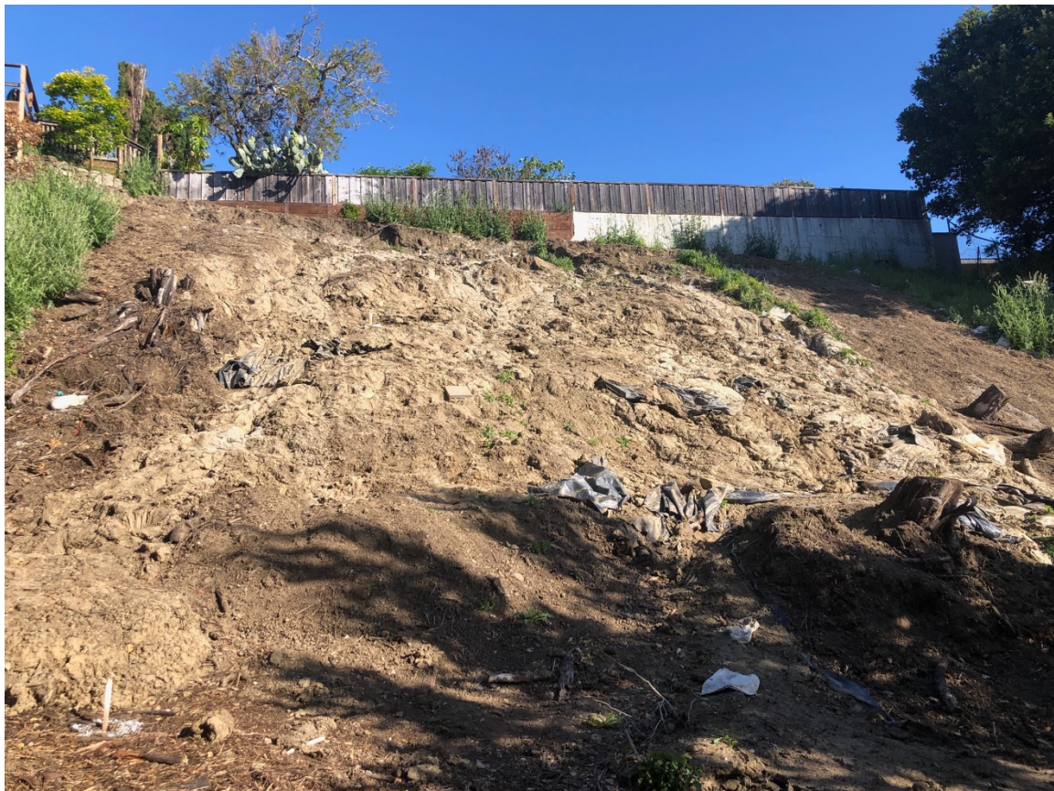
Photo 4: View towards the northwest of the slide area from the toe of the slide. Note that the steel I-Beam and wood lagging retaining wall behind 2839 Arguello Drive (design plans not reviewed) is visible below the fence and to the left of the white concrete retaining wall.
